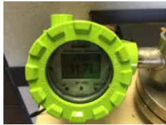
Photograph No. 1 Enclosure – Front
